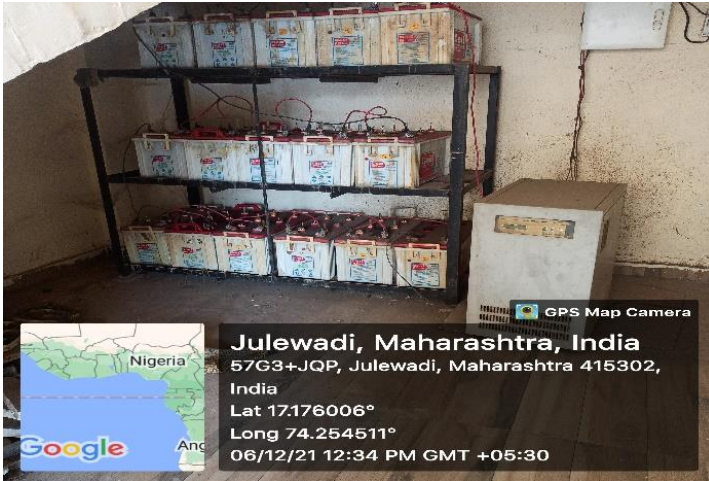
Battery in office
